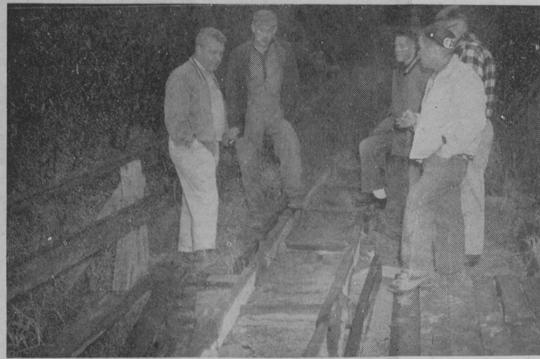
A WORK BEE was held Sunday afternoon at Silver Valley. James Campbell, winter sports committee president, is shown at left discussing the rebuilding of a new bridge for the return toboggan slide. Another bee will be held this Sunday and volunteers are needed to get the park ready for the coming season.—Tawas Herald Photo.
