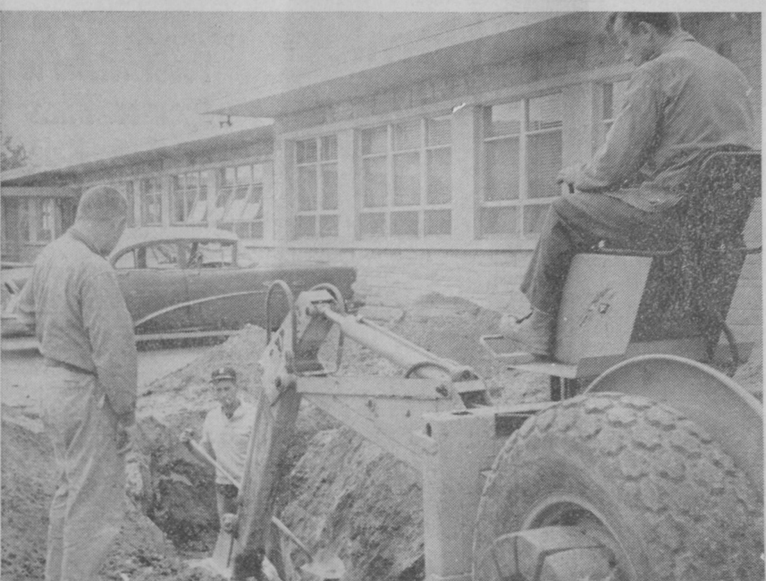
WORK STARTED last Wednesday on a 32 by 52-foot addition to the Iosco County Building. William Gregory, general contractor of Bay City, is shown at left while footings were being dug. The addition will house a new meeting room for the board of supervisors and is to be completed by late October. The addition is located on the north side of the building.—Tawas Herald Photo.
