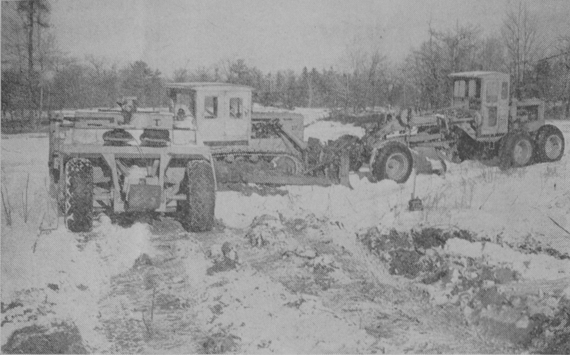
CONSTRUCTION has started on relocating the road on Tawas Point for the new state park. This picture shows earth-moving equipment which is being used on the project. Conservation department officials said the road's new location would allow better utilization of the property for park purposes. Ownership of the old road has reverted to the state.—Tawas Herald Photo.
