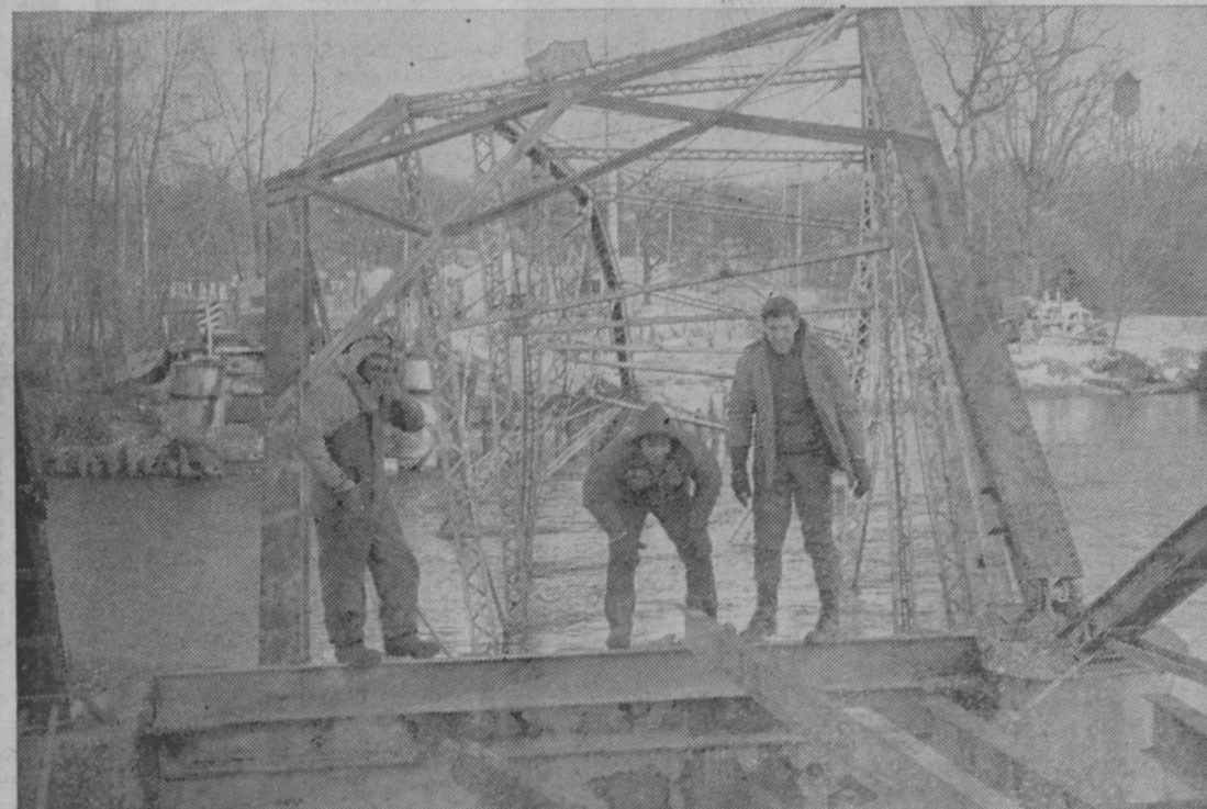
THE OLD IRON BRIDGE spanning the AuSable River at Oscoda was pulled off its piers Saturday afternoon as preparations were made to remove the structure. Gallagher and Company, Incorporated, of Novi is contractor for the Isoco County Road Commission. A new $150,000 bridge is to be constructed there next spring. The project is being financed jointly by federal aid from the United States Bureau of Public Roads, Isoco County and Townships of Oscoda and AuSable. The old one-lane bridge had served for more than 60 years.—Tawas Herald Photo.
