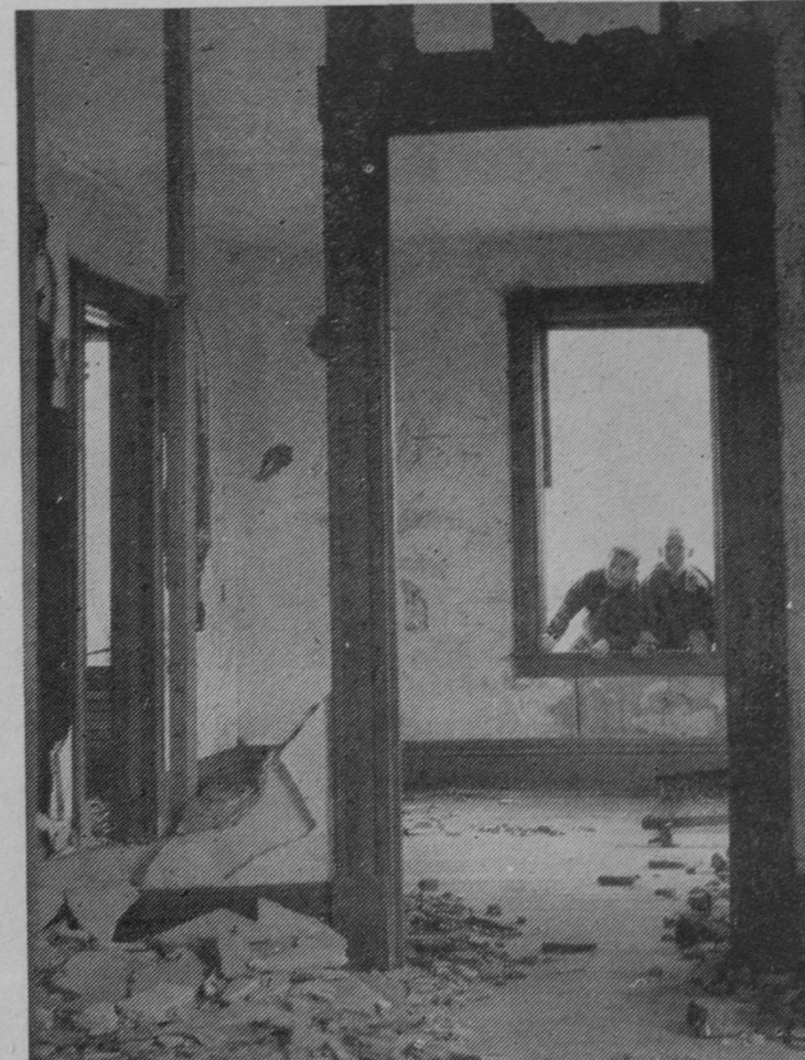
VANDALS have gutted the interior of the old coast guard light house located on the north tip of the island. This picture was snapped during a recent inspection trip by coastguardsmen from Tawas Point.—Tawas Herald Photo.
