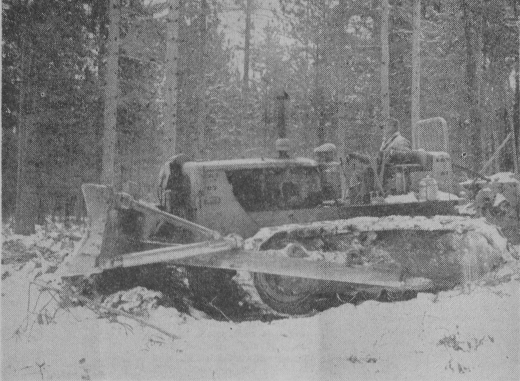
CONTRACTORS for Michigan Consolidated Gas Company are presently at work clearing a right-of-way line for the gas main north to Alpena. This bulldozer was at work Friday west of the Arthur Leitz residence in Baldwin Township.—Tawas Herald Photo.
