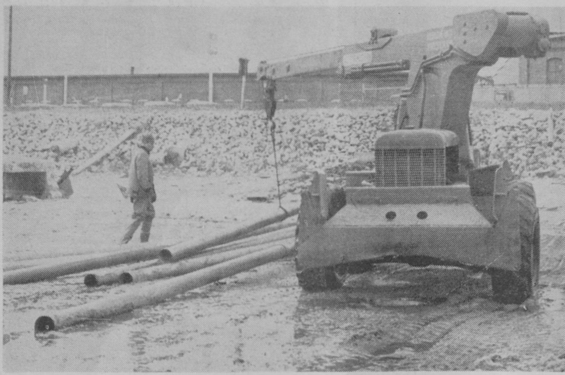
AN OLD WATER LINE which once pumped water from Tawas Bay for use in steam boilers and locomotives of the Detroit and Mackinac Railway was removed from the lake bottom last week. Low water in the bay has exposed numerous old water lines and breakwalls and this was the first to be removed. Waves once splashed against rocks protecting US-23 in the background. —Tawas Herald Photo.
