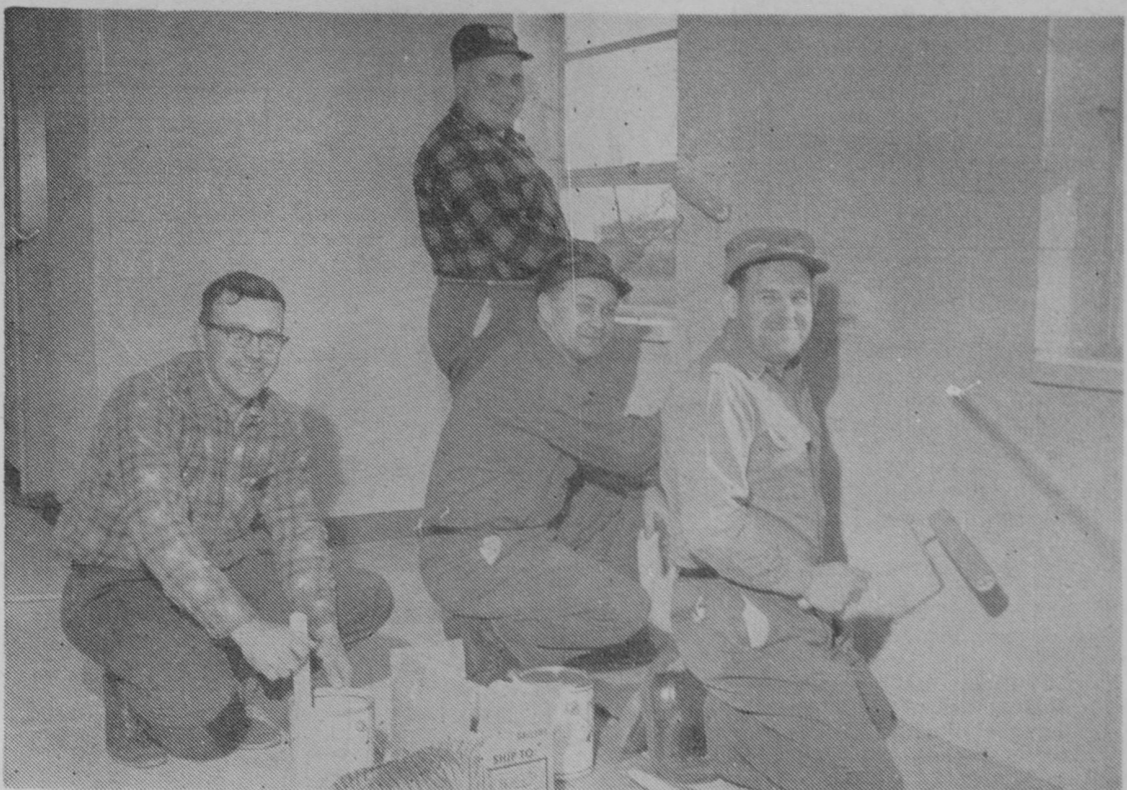
FIRE CHIEF James Mann, left, and members of the Plainfield Township Fire Department are shown painting the department's new fire hall at Hale. Others are John Hendrickson, Lloyd Springsteen and James Schroeder.—Tawas Herald Photo.
