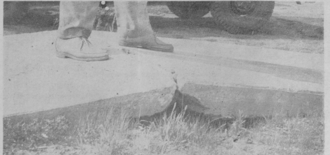
THE SUN was mighty hot Tuesday and this buckled sidewalk in front of Ottawa Equipment Company, Tawas City, attests to that fact. It is believed that the massive slab of concrete in front of the building expanded, forcing the sidewalk to buckle.—Tawas Herald Photo.
