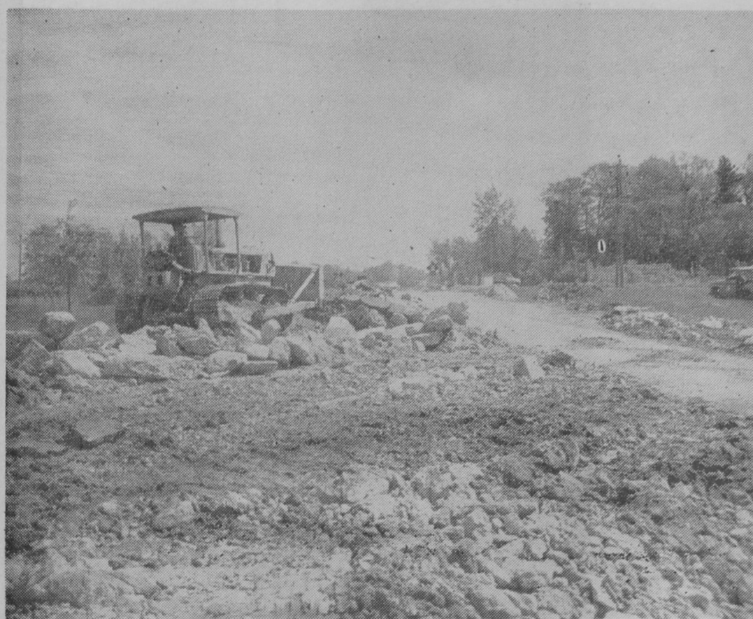
SOUTHBOUND LANE of US-23 at the Alabaster curve is being torn up during current construction work by contractors for the state highway department. Concrete in that area had shattered during recent years and is to be replaced. The highway from the Tawas City limits to the Arenac County line is being widened and is to receive a blacktop surface.—Tawas Herald Photo.
