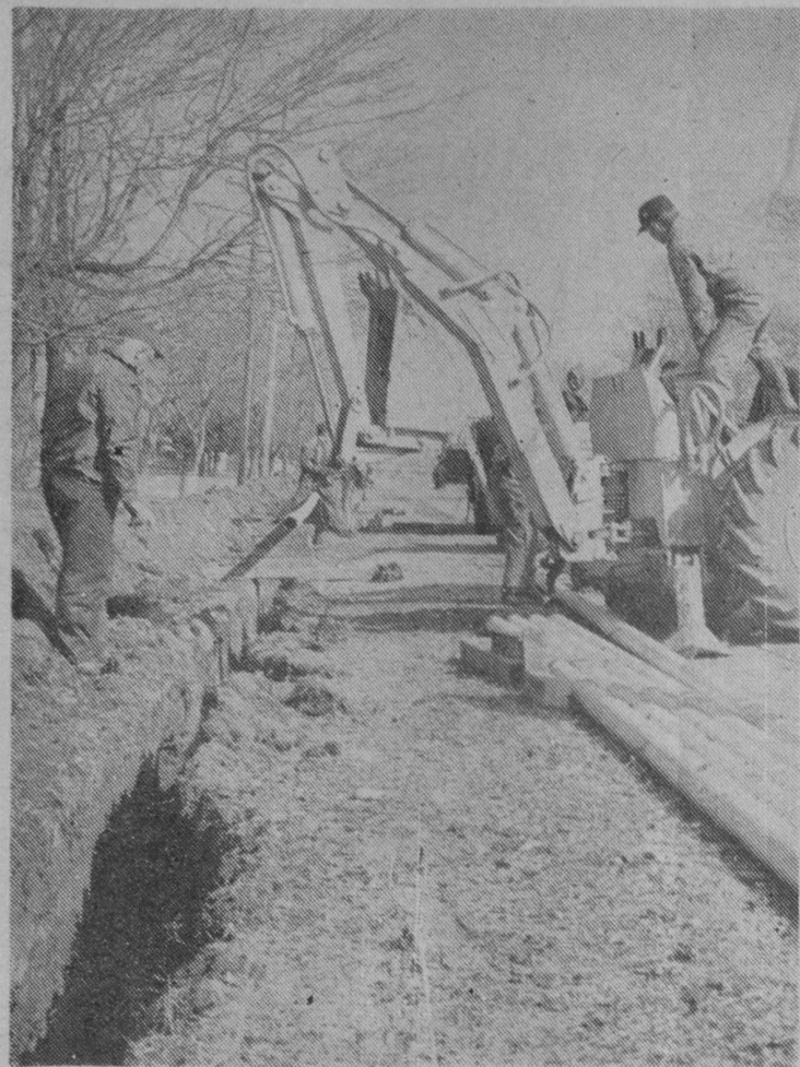
CONSTRUCTION was started Tuesday morning by contractors for Michigan Consolidated Gas Company on distribution mains to serve the Tawas. The above picture was snapped along Fifth Avenue in Tawas City. Scheduled completion date is August 1.—Herald Photo.
