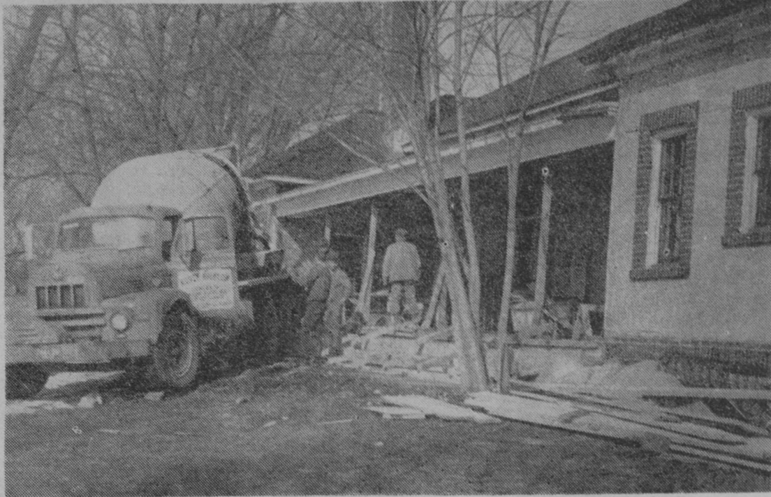
WORKMEN are pictured here pouring new concrete steps for the south porch of the East Tawas Community Building, now being remodeled by the Eckstein Construction Company. This work is part of a $35,000 improvement program at the East Tawas Park, obtained earlier this year from the Michigan Department of Conservation. The change was brought about by construction of the new state park on Tawas Point.—Tawas Herald Photo.
