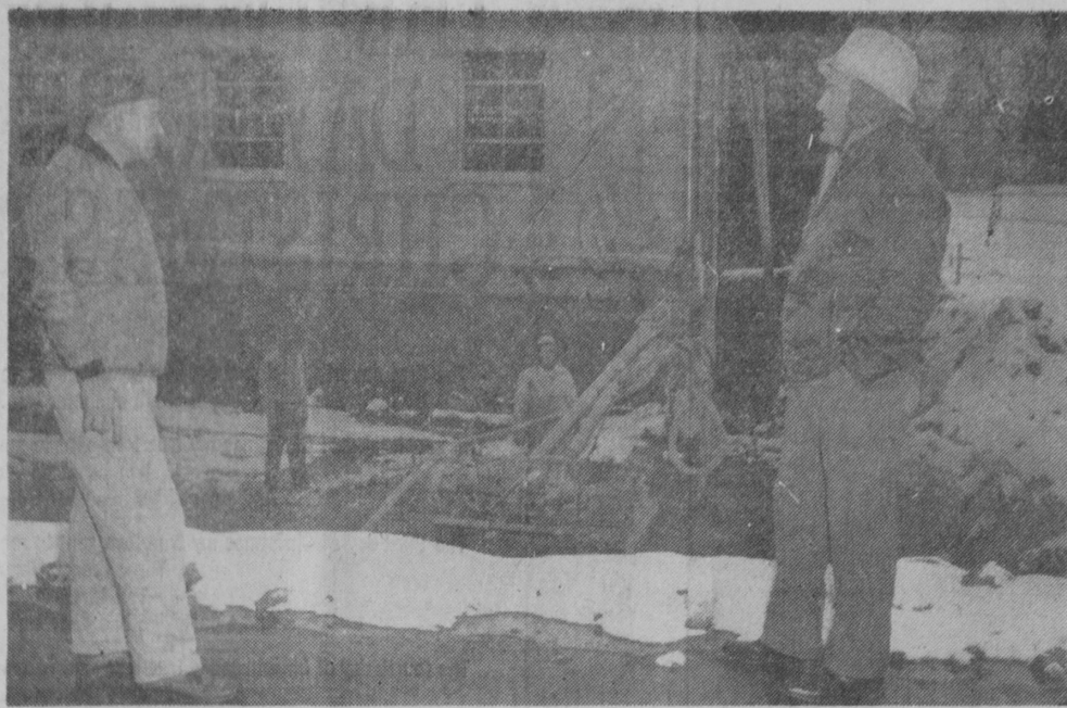
LOOKING OVER the start of expansion of the Whitestone Point Pumping Station at Saginaw-Midland Water Supply are William Grebe, right, operations and maintenance foreman for the water system, and Michael Schwartz, left, owner of Power Blasting Company, Incorporated, Luke Servant, project superintendent, stands below at left.—Tawas Herald Photo.
