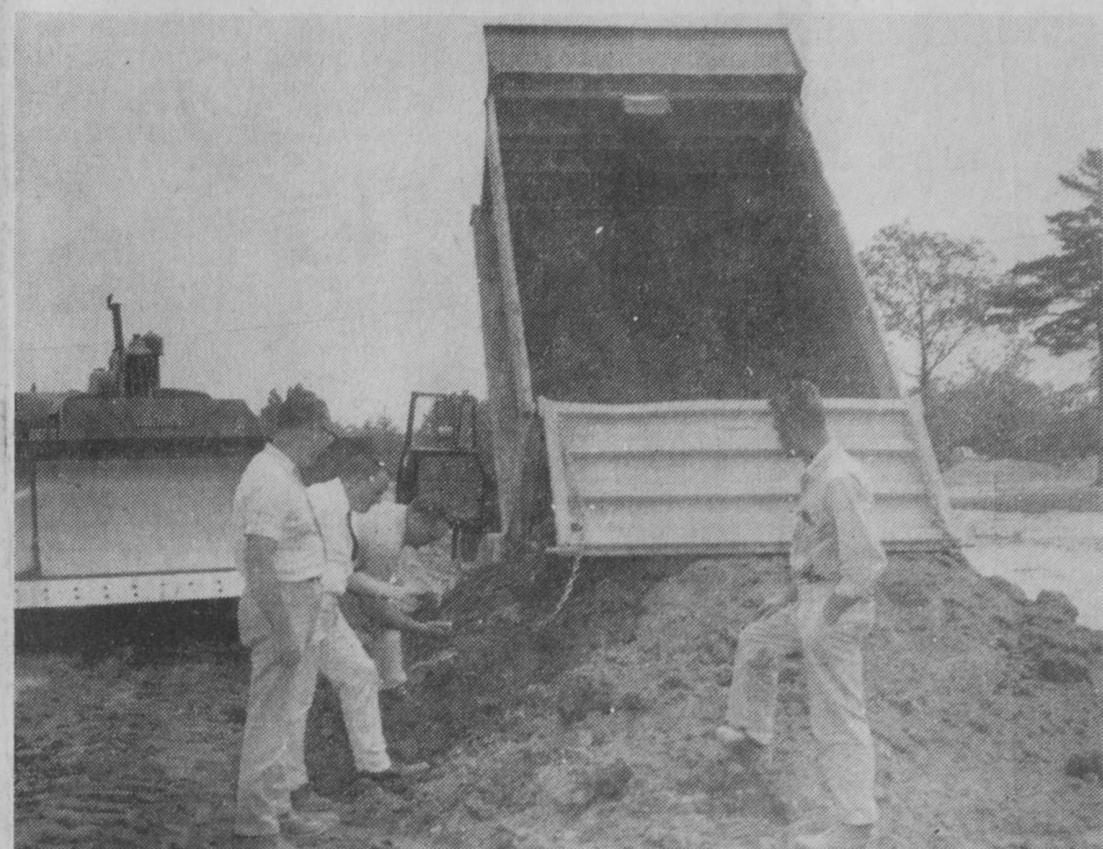
TOP SOIL from an old farm on Meadow Road has been donated by National Gypsum Company to the Michigan Department of Conservation for use at Tawas Point State Park. Watching the spreading of one load of the 5,000 yards of top soil to be moved are, from left: Contractor Jack Doherty, Richard Harris of National Gypsum Company, Park Supervisor A. Ray Prosch and Contractor Lyman Gerst.—Tawas Herald Photo.
