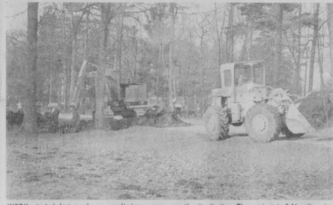
WORK started last week on preliminary construction for widening and resurfacing US-23 through Tawas City. The above picture shows equipment of T. A. Forsberg, Okemos, contractor for the state highway department, removing trees and constructing storm drains near the south city limits. The project is 2.46 miles in length and Forsberg's bid was $333,175. Curbs and drains are to be constructed and the highway will receive a top of bituminous asphalt. The project is to be completed by next fall.—Tawas Herald Photo.
