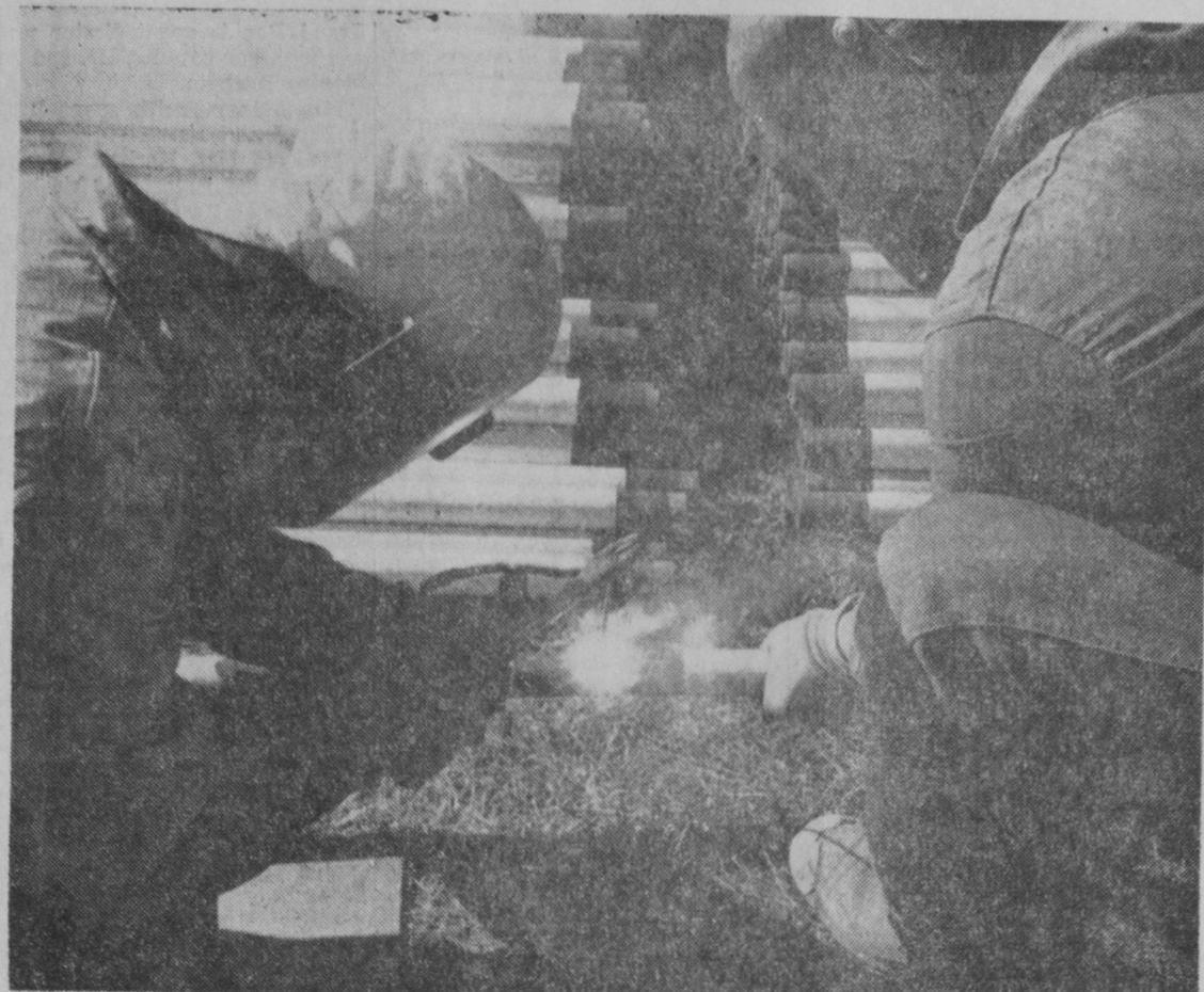
WORK WAS STARTED Wednesday morning by Welded Construction Company, Clare, on Michigan Consolidated Gas Company's pipeline expansion project to serve the community of Hale. The pipeline is to be extended north from M-55 about 6 1/2 miles to Hale and the main is to be extended west to Putnam Road and east on Main Street within the village. Ground was
