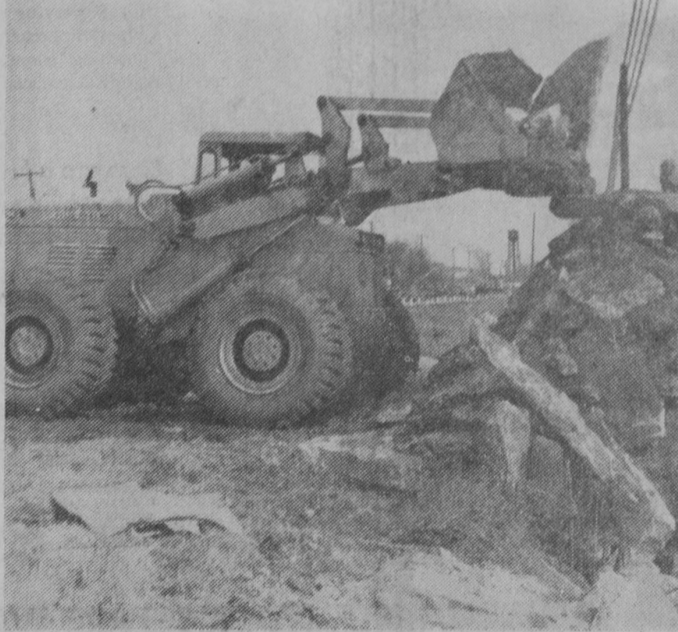
BROKEN CONCRETE is pushed toward the lake side of US-23 in the above picture. The project is 2.46 miles in length. Widening and resurfacing will cost $333,175.—Tawas Herald Photo.
