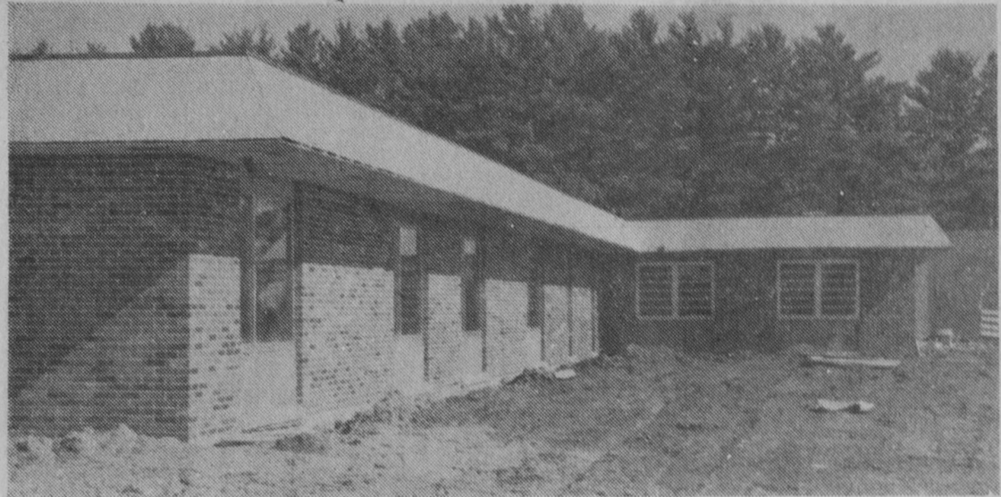
CONSTRUCTION on the new Iosco County Medical Facility is progressing rapidly and the new home for the aged is scheduled to be completed by May 24. The new facility is being financed by a $300,000 general obligation bond issue approved by Iosco voters and a $250,000 Hill-Burton federal grant. This picture shows construction on the south side of the building.—Tawas Herald Photo.
