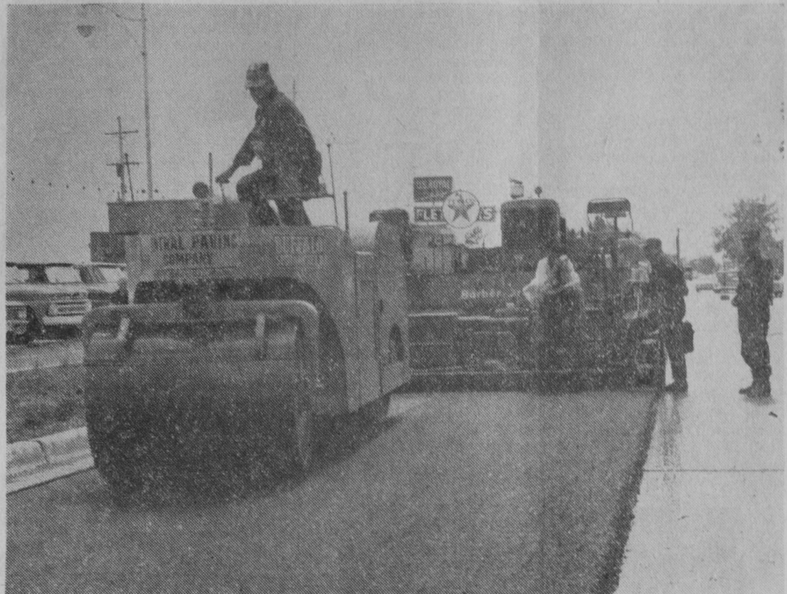
WORK on applying the first coat of blacktop on US-23 was completed last Friday between the city limits at East Tawas and Mathews Street in Tawas City. Construction began Monday on the highway south of Mathews Street. Following the initial layer of blacktop, Central Paving Company, West Branch, will return to the east city limits and begin a final layer on the four-lane highway.—Tawas Herald Photo.
