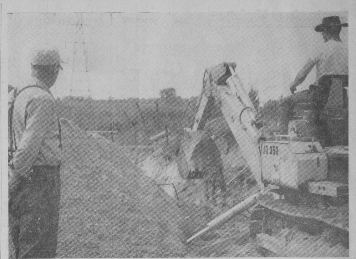
WORK was started last spring and completed during the summer on a new sewer system for a trunkline main in the above photo.—Tawas Herald Photo.
