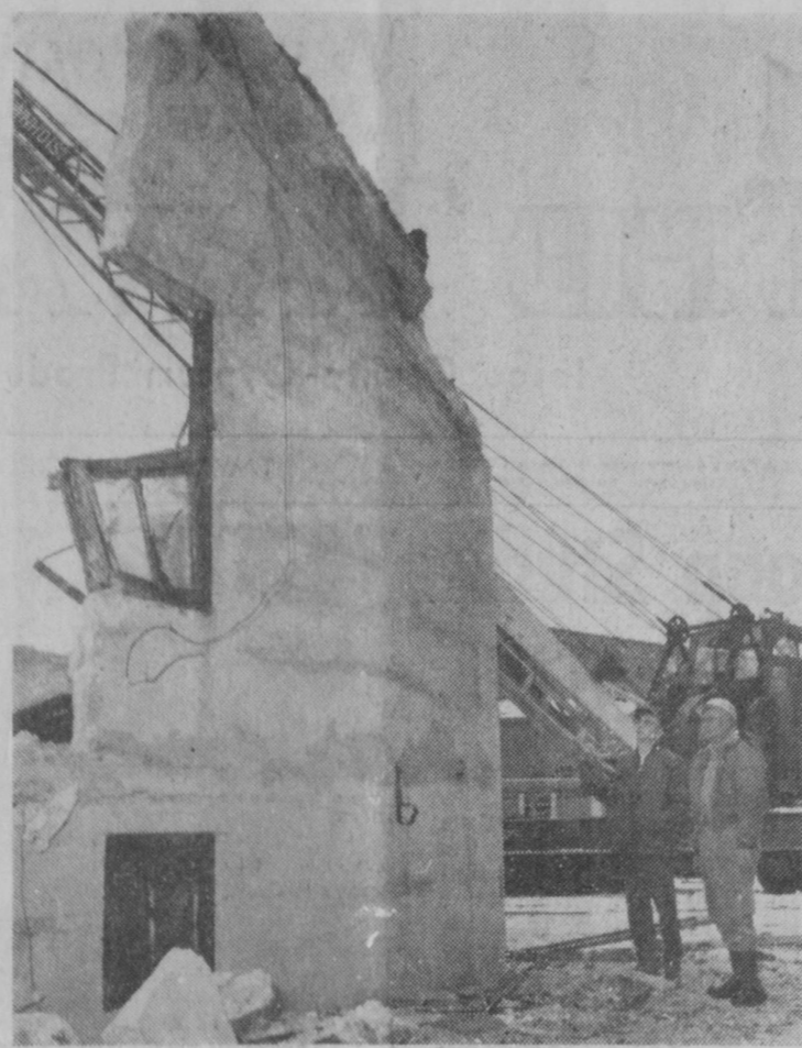
ANOTHER RELIC of the steam locomotive era was removed from today's scene when the Detroit and Mackinac Railway demolished an old concrete building which once served to store locomotive lubricants at the Tawas City yards. The building was constructed in May 1905. Maintenance Supv. J. E. Dougherty, left, and Clark Tanner are shown inspecting one wall of the building before it fell before blows of the dragline in the background.—Tawas Herald Photo.
