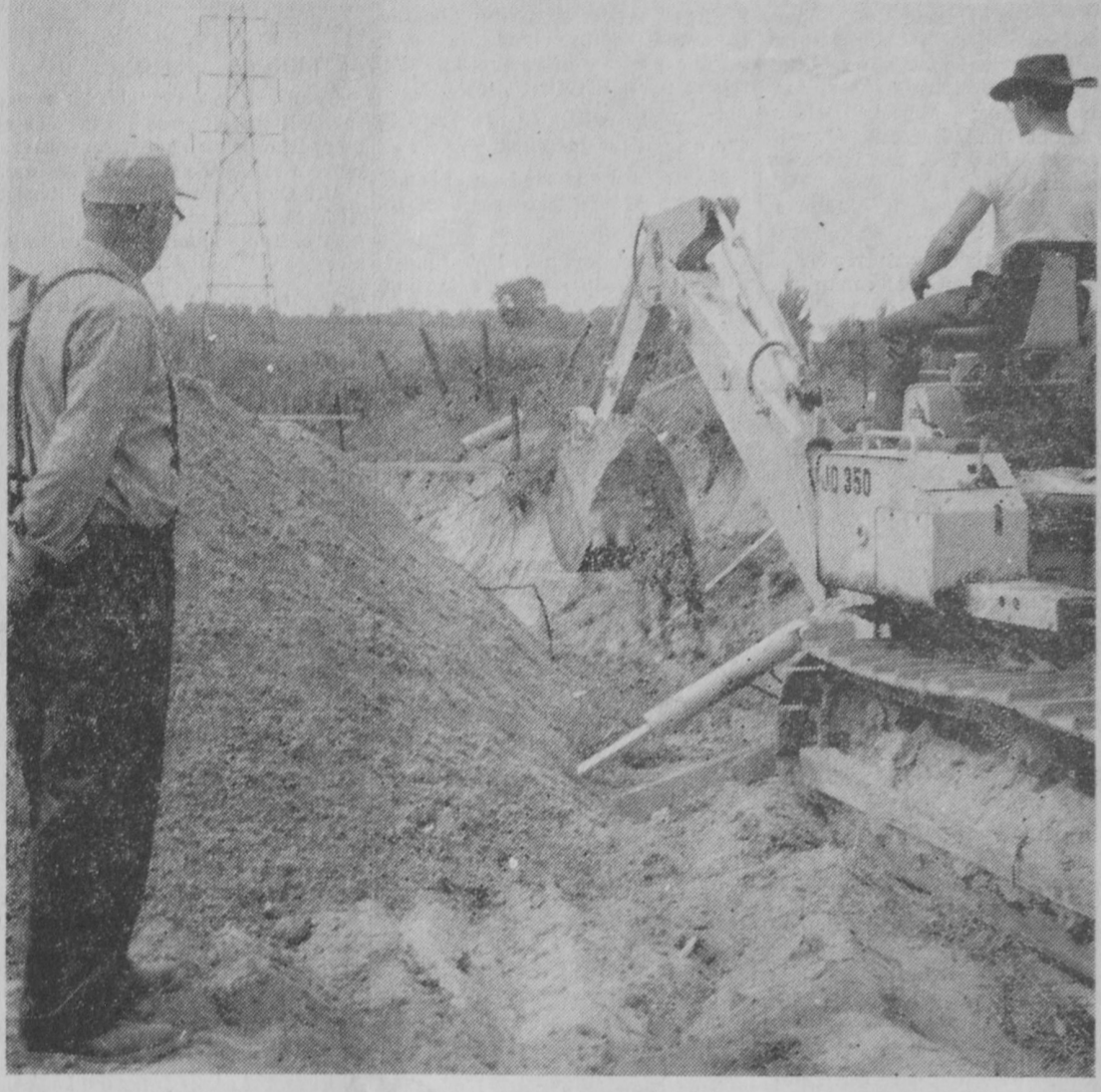
GROUND was broken last week on construction of a $48,000 sewer system to serve Hale. Shown at left in the above picture is Lawrence Shaum, inspector on the project for Plainfield Township. Operating the backhoe machine is James Mann.—Tawas Herald Photo.
