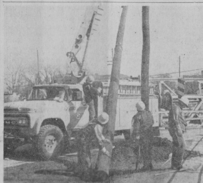
CONSTRUCTION of a new electrical power line through Tawas City is now under way by Consumers Power Company. This picture shows workers setting a pole near the Mathews Street bridge. The line replaces one along Court Street which is nearly 30 years old.—Tawas Herald Photo.
