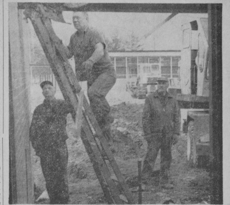
WORK started last week on construction of five new classrooms at Tawas Area High School. Employees of O. S. Rose Construction Company, general contractor, are shown above Monday morning as an overhanging entrance was removed from the southwest corner of the building.—Tawas Herald Photo.
