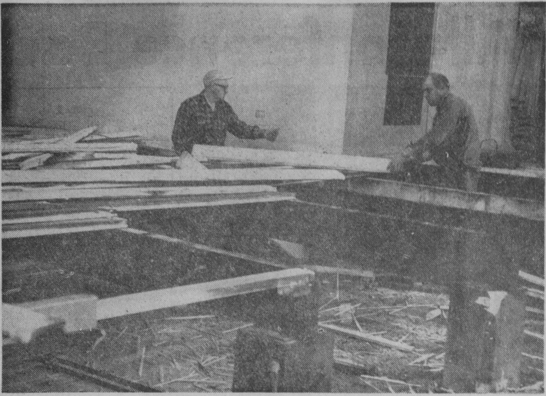
FIRE CAUSED extensive damage to Tawas Area High School Auditorium last Wednesday morning. Faulty electric wiring is believed to be the cause of the blaze under the stage. Workers are shown removing charred timbers in the above photo. Although some smoke damage was caused, the fire was brought under control before spreading further.—Tawas Herald Photo.
