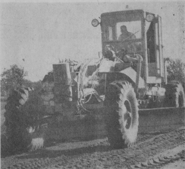
EQUIPMENT of the losco County Road Commission is pictured above as construction was under way on Esmond and Londo Lake Roads in Plainfield Township last Wednesday.—Herald Photo.
