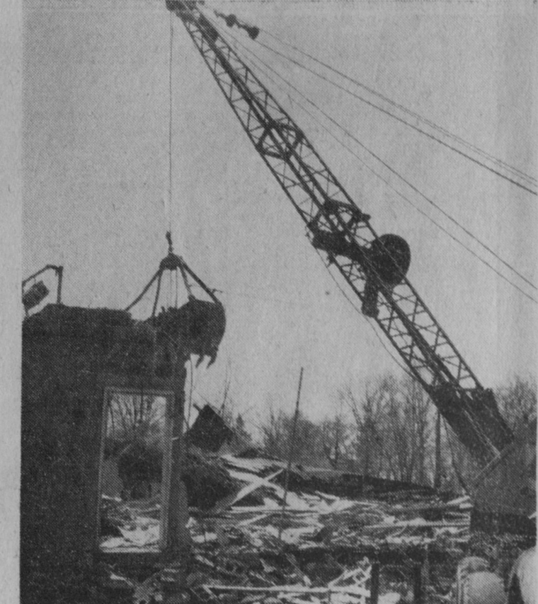
DEMOLITION of the old Bayview Restaurant building at East Tawas is nearly complete. Built by the late Nicholas Pappas in 1931, the property has been purchased by the owners of Norman's Department Store, West Branch, and a new 41 by 80-foot building is to be constructed for a new apparel store.—Tawas Herald Photo.
