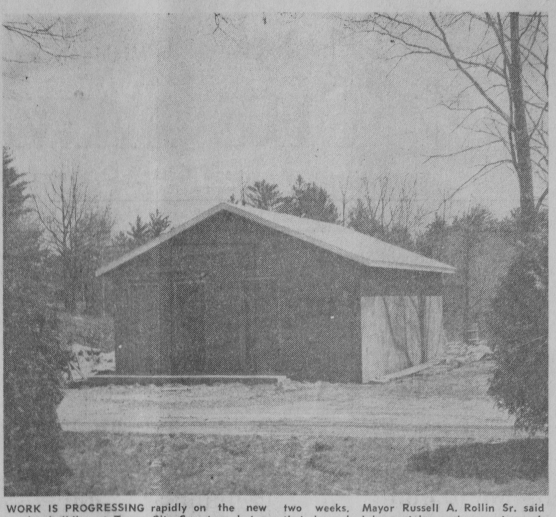
WORK IS PROGRESSING rapidly on the new service building at Tawas City Cemetery, but a city official noted Monday that considerable vandalism had taken place there during the past two weeks. Mayor Russell A. Rollin Sr. said that doors had been stolen and concrete work had been damaged. Tawas City Police Department is investigating.—Tawas Herald Photo.
