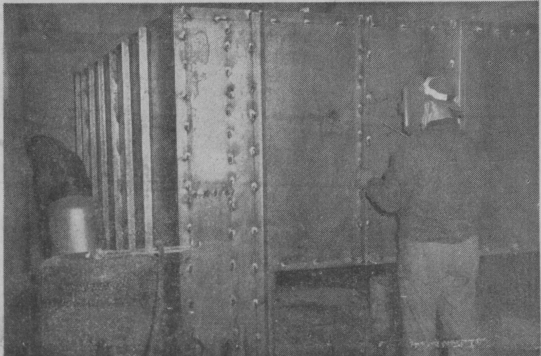
CONSTRUCTION has progressed rapidly on replacing the frame sawdust drying building which was destroyed by fire last week at Tawas Industries, Incorporated. The top photo shows progress as of Monday on the concrete block building, while the lower photo shows a workman welding the new steel sawdust bin. Equipment is being installed this week.—Tawas Herald Photos.
