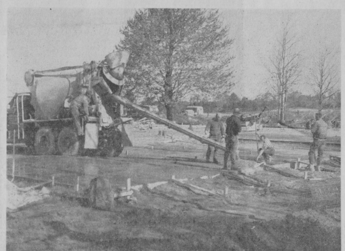
WORKMEN began pouring a concrete slab for a new industrial building at Hale last week. Located east of Hale on Esmond Road, the building is to house a new plant which will manufacture archery equipment. The building is owned by Hale Development Corporation.—Tawas Herald Photo.
