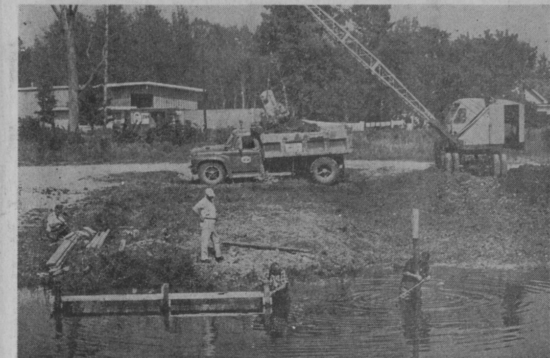
PROGRESS on Tawas City's second boat launching ramp on Tawas River is pictured above Monday morning. A third double ramp is planned for the future. New parking facilities are to be located to the left of the building in the background.—Tawas Herald Photo.
