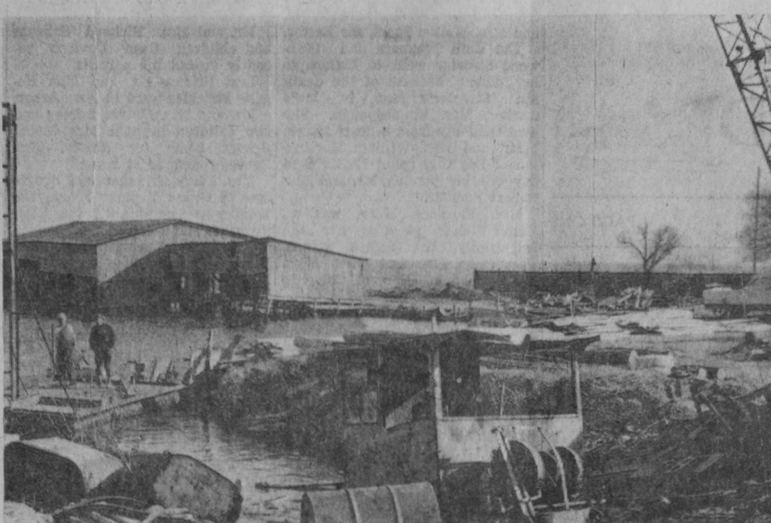
WORK STARTED last week on constructing a new boat basin at the Tawas River mouth for Coho City Marina, located on the west side of the river. A pile driver is being used to build a retaining wall around the basin. Gasoline storage tanks were installed on Friday.—Tawas Herald Photo.
