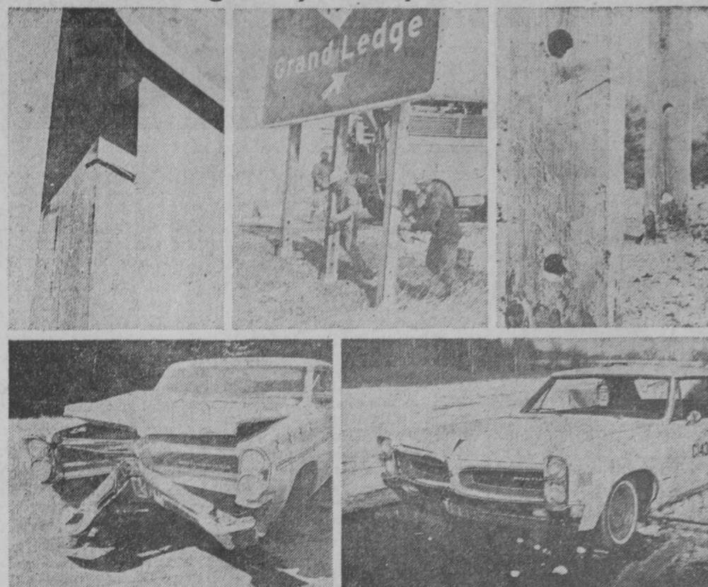
A NEW SAFETY FEATURE on state highways in Michigan is the use of wooden breakaway sign supports, center, in place of steel supports. Now being installed at select locations, the wooden supports have a slot near the base of the sign, upper left, and two holes just above ground level, upper right, to insure the breakaway effect. Two vehicles, each traveling 60 miles an hour, proved the value of the breakaway supports in tests at the General Motors Proving Grounds. The one at lower left hit a steel support. The other, at lower right, hit a breakaway support and had only minor damage. (Department of State Highways photos).
