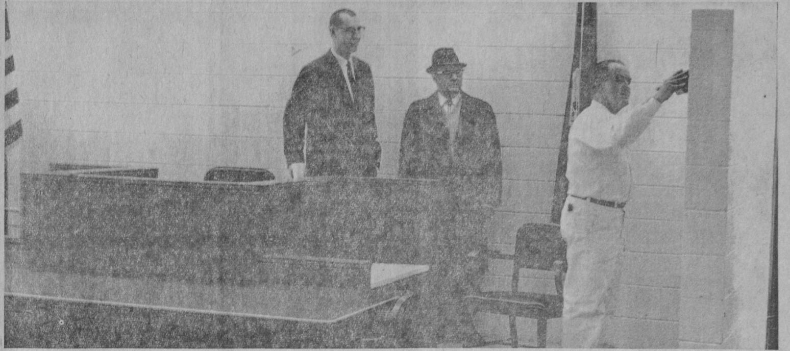
FINISHING TOUCHES were being put on the new district court room Tuesday morning by Walter Nelson, right, painting contractor, Judge Richard Ernst, left, and Robert Foster, a member of the county board of supervisors, survey the work. The board of supervisors is to meet in the room today. The room formerly had been used exclusively by the supervisors. Two offices were constructed for the court.—Tawas Herald Photo.
