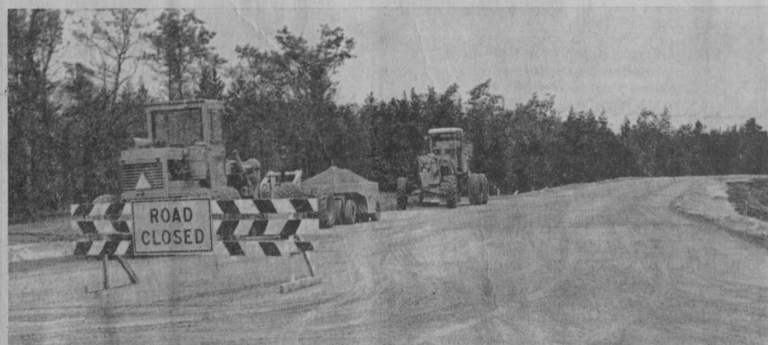
WORK is progressing on rerouting of 1.7 miles of River Road at the Lumbermen's Monument. This construction is being handled by a contractor for the Department of State Highways. Scheduled to be completed November 1, the new route has been moved several hundred yards south of the monument in order to provide better parking and expand facilities.—Tawas Herald Photo.
