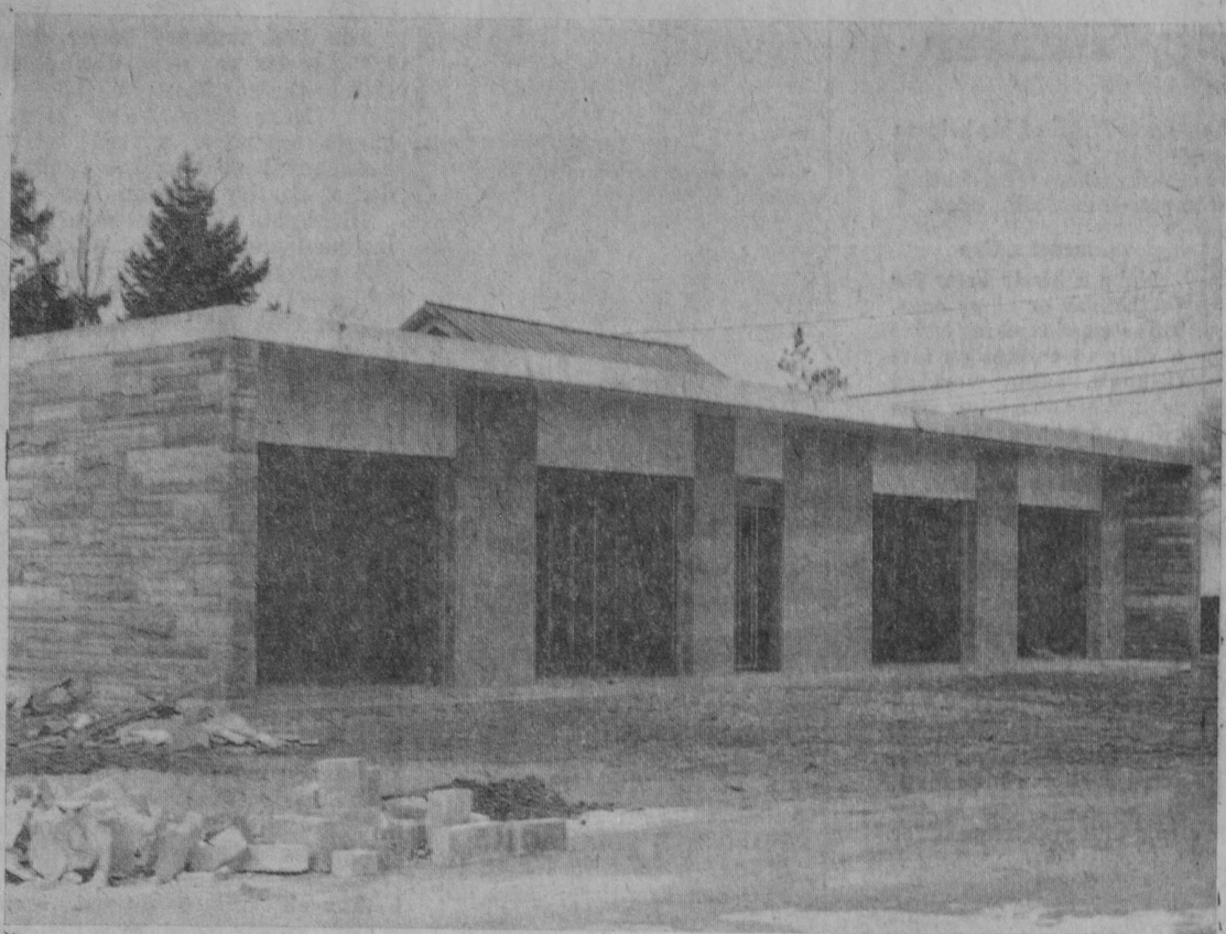
PROGRESS on construction of a new garage at the Isosco County Jail is pictured above. Contractor for the $20,387 structure is Don Reed Construction Company, Lincoln. The new 30 by 60-foot garage is being constructed to conform with lines of the jail and county building. Stone on the front of the building matches that on the jail and county building. It is to be used for storage of sheriff's department vehicles and boats used in water enforcement patrols.—Tawas Herald Photo.
