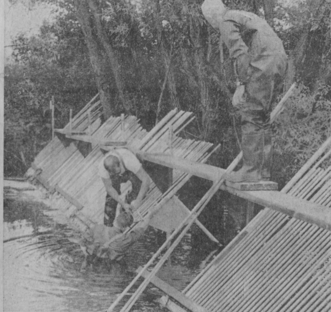
WHEN COHO began to pour through an open weir in the Tawas River Monday, a crew from the Michigan Department of Natural Resources was on hand Tuesday morning to close the gap. The crew installed signs prohibiting fishing in the river below the weir.—Tawas Herald Photo.
