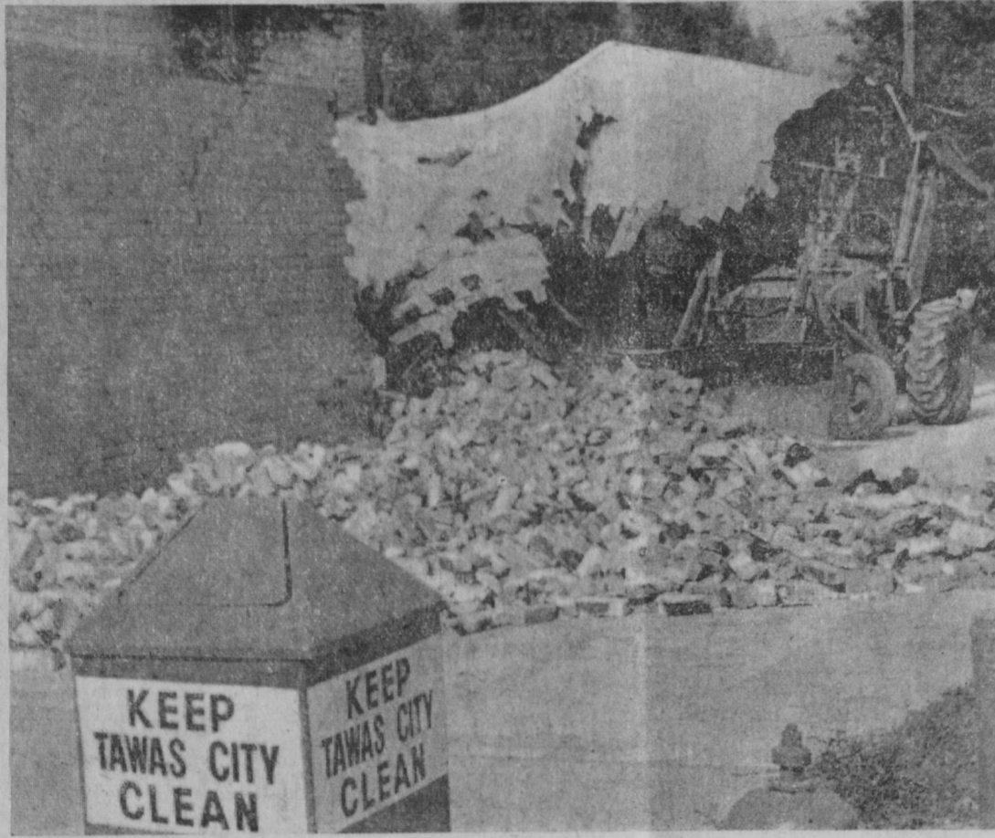
WORK WAS STARTED last week on removal of the fire-damaged Schultz Hardware Building in Tawas City. Contractor for the project is Roy Newman Sr., M-65, near Hale. The building had been hit by a fire nearly one year ago.—Tawas Herald Photo.
