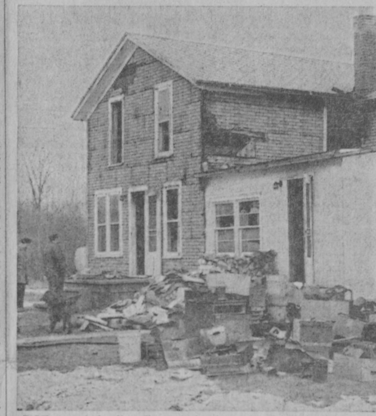
FIRE gutted the first floor of this house on Ruell Road Monday night and caused extensive damage to the upper floor. Tawas City firemen battled the fire for several hours, then were called the next day to extinguish another blaze.—Tawas Herald Photo.
