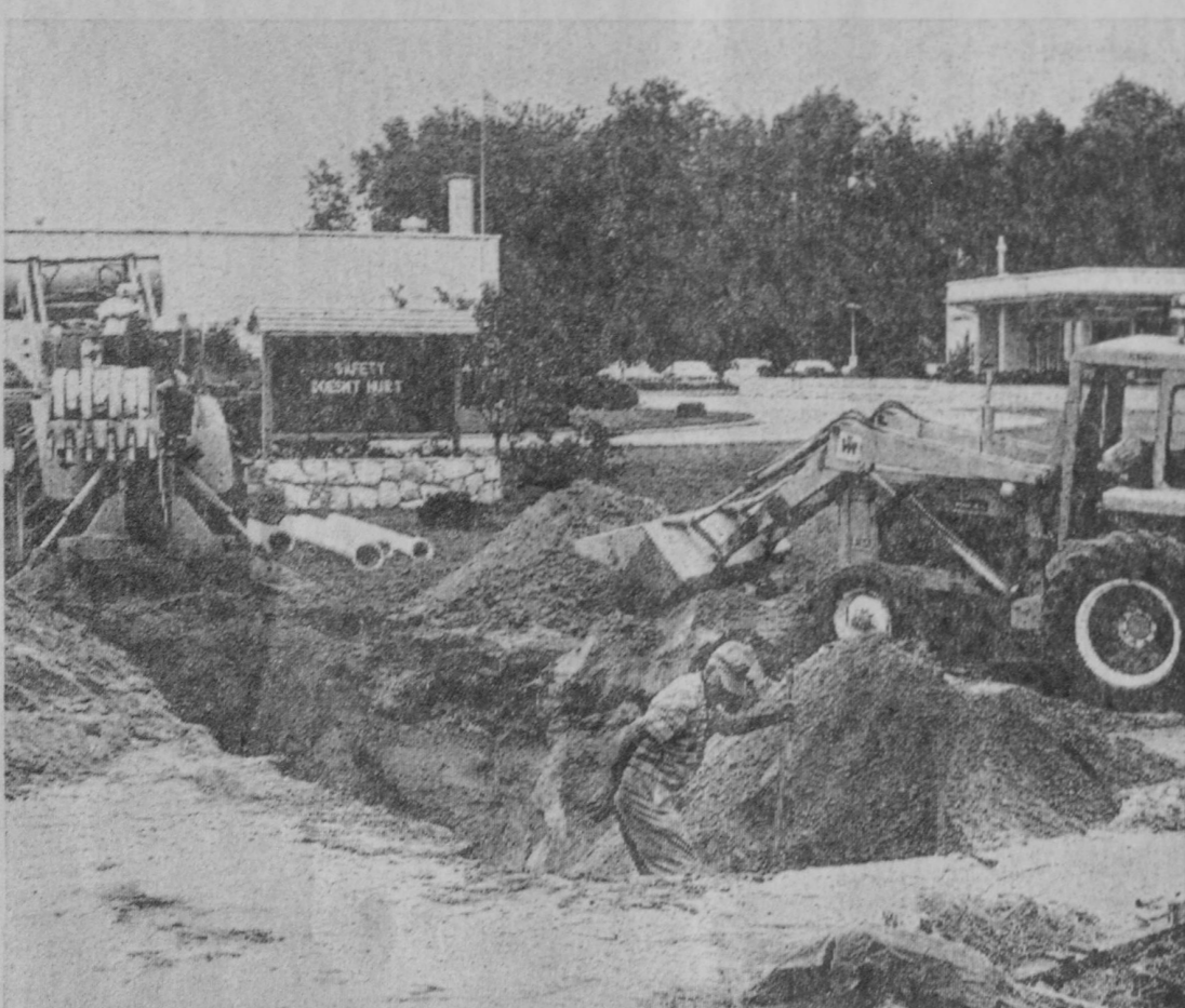
PROGRESS on construction of a new water main to serve expansion at Tawas Hospital is pictured above. The work is being performed by the Tawas
