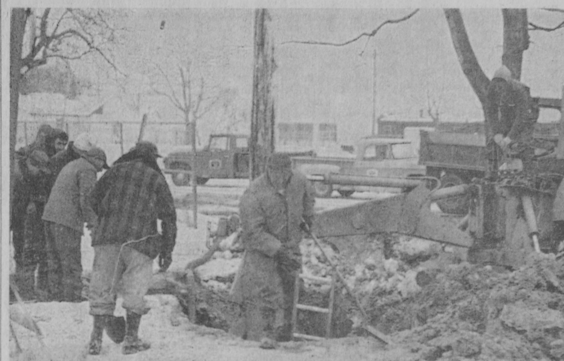
COLD WEATHER has provided added problems for the Tawas City Department of Public Works. A water main cracked last Tuesday night and repairs were made to the line Wednesday, but not
