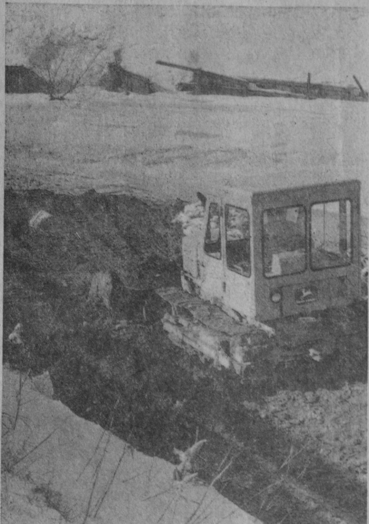
WORK STARTED Tuesday on building a temporary earthen dam in the Tawas River. The dam will facilitate repair to a broken water main under the river.—Tawas Herald Photo.
