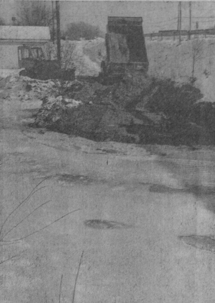
LOOKING east across the river at the US-23 bridge, a city truck dumps sand on the river bank.—Tawas Herald Photo.
