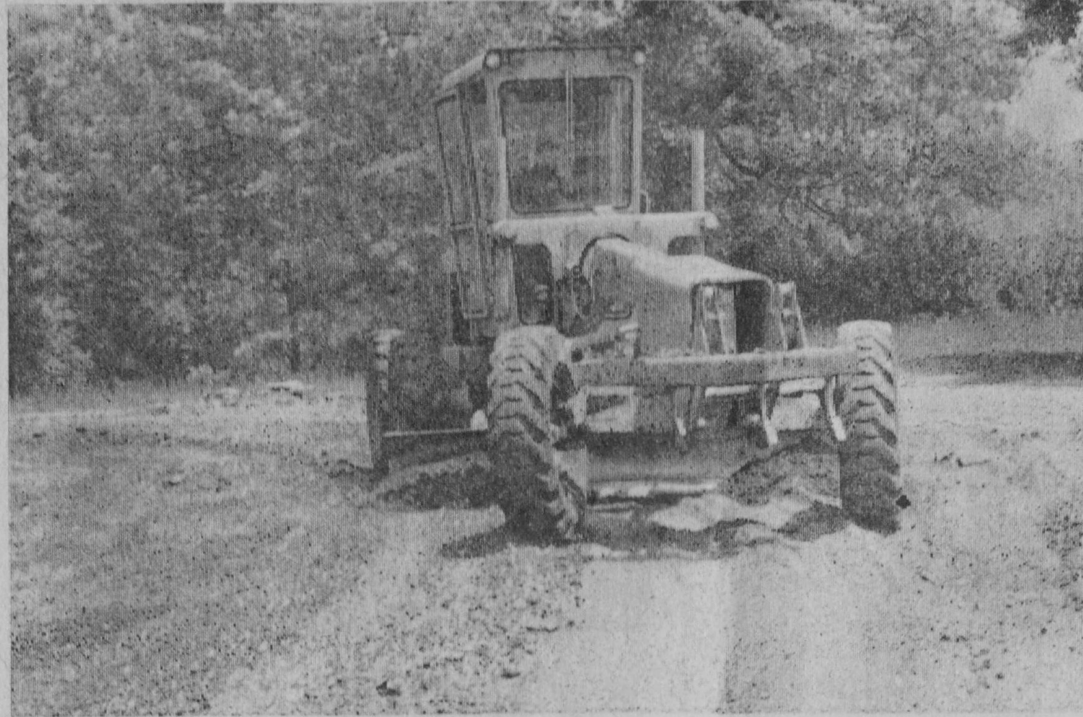
WORK STARTED Monday on the initial phase of Tawas City's $18,000 street construction program for 1970. Yockey Construction Company, contractor began preparing several streets for seal coating with a soil stabilization process. This is the same type of construction used on First Street five years ago. The bituminous seal coat is to be applied next week.—Tawas Herald Photo.
