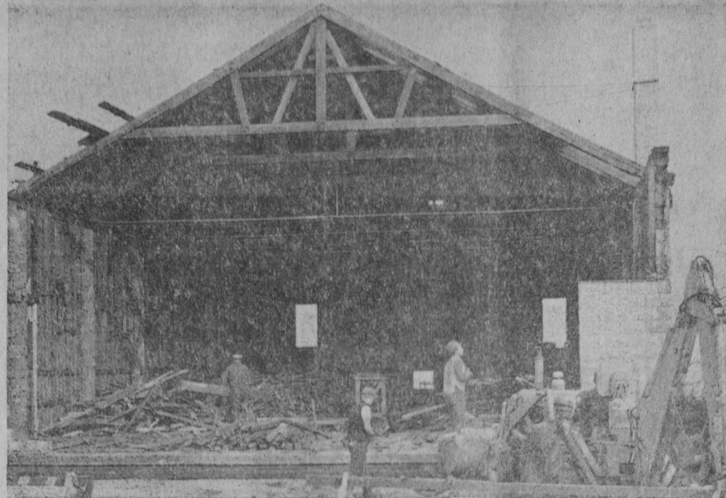
PROGRESS on removing the old Bay Theatre building in Tawas City is pictured here. Being removed for a street level parking lot to serve Keiser's Drug Store, oldtimers say that when constructed in the 1920s, it was the opinion of some that the building had faulty engineering and would soon cave in. Ice sliding off the roof during the showing of a silent picture one night touched off a near panic, but the building has been standing for nearly 50 years.—Tawas Herald Photo.
