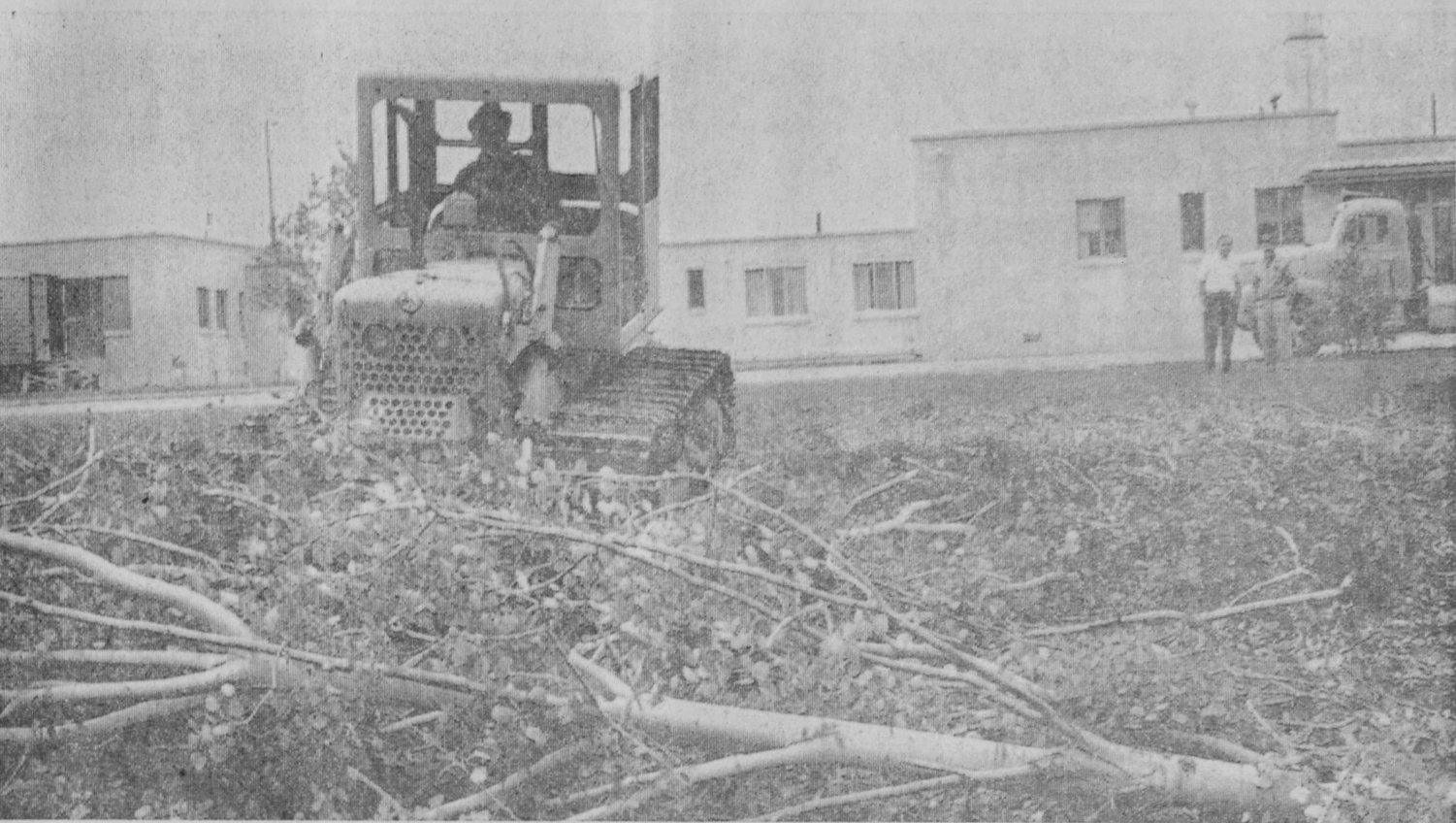
FOLLOWING official ground breaking ceremonies two weeks ago, work began Monday on the actual clearing of the site for an addition to Tawas Hospital. This picture was snapped looking south toward the hospital. A number of trees were removed and the site is to be brought to grade.—Tawas Herald Photo.
