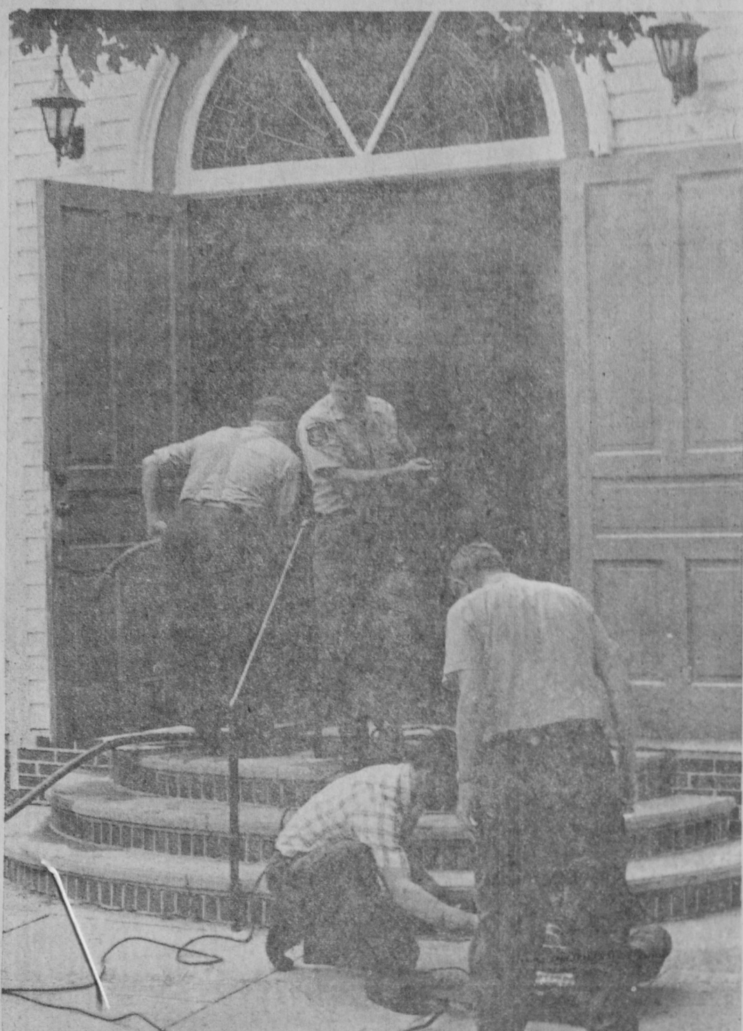
FIRE CAUSED extensive smoke damage Friday noon to Emanuel Lutheran Church, Tawas City. The blaze started in a storage room under a stairway leading to the choir loft and filled the building with smoke. According to Fire Chief James Lansky, heat caused a window to blow out at the southwest corner of the church and two boys
