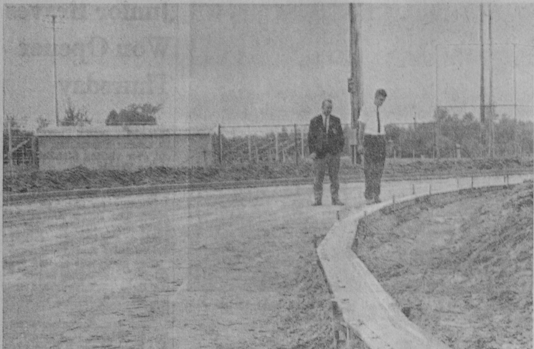
WORK STARTED last week on construction of a new all weather track at Tawas Area High School. The new track is to be ready for use next spring. The project is being financed through a revenue bond issue. Looking over progress above are Coach Robert McDonald and Bill McIntosh, athletic director.—Tawas Herald Photo.
