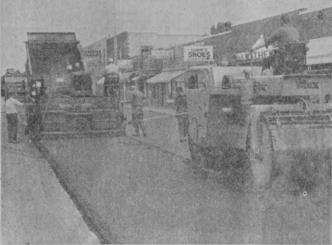
WORK STARTED early Wednesday morning on reconstruction of two blocks of the Newman Street business district at East Tawas. The project of laying a new surface of plant mix asphalt was completed in one day. Work on the project, which was a tremendous improvement to the street, is pictured above.—Tawas Herald Photo.
