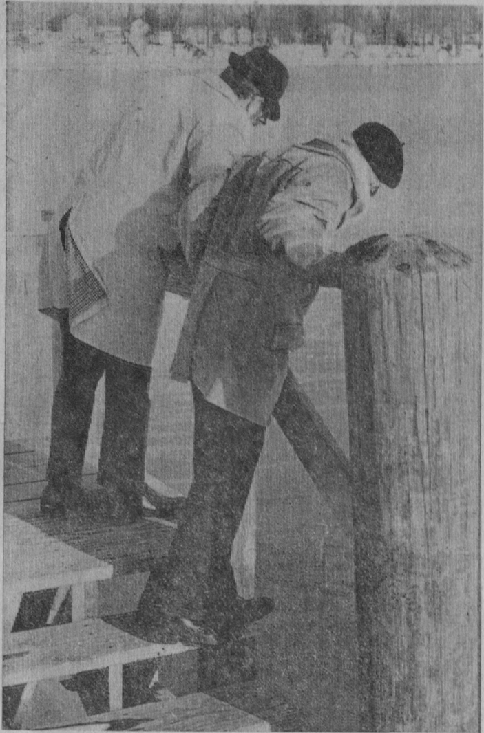
HUGE PILINGS like the one in the foreground are beginning to show deterioration at the Michigan Waterways Commission Dock. Leaning over the rail at left to get a closer look is Keith Wilson, director of the waterways commission.—Tawas Herald Photo.
