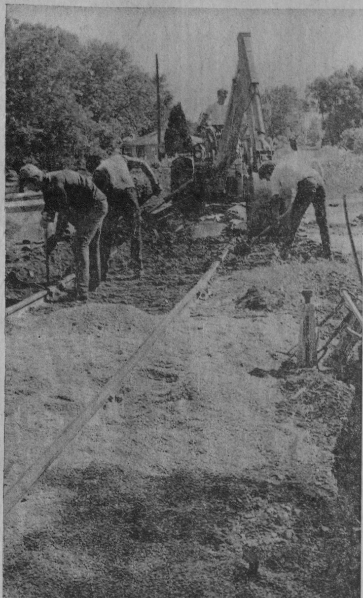
WORK RESUMED TUESDAY on rebuilding the roadbed of the Detroit and Mackinac Railway Company through Tawas City. Tracks are being raised and leveled in some areas and heavier rails are being installed. This picture shows the road crew at work on the Whittemore Street grade crossing.—Tawas Herald Photo.
