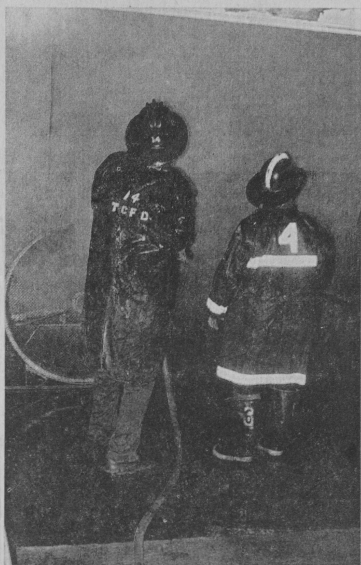
A FAULTY ELECTRICAL CIRCUIT was blamed for Thursday night's fire which caused extensive damage to the sawdust drying building of Tawas Industries, Incorporated, Tawas City. Work on repairing the building was commenced the next day and the drying operation is expected to resume production by Wednesday (today). Sawdust is used by the firm in the manufacture of auto-
