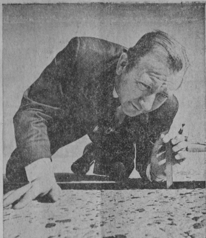
STATE REP. THOMAS FORD OF GRAND RAPIDS, demonstrates on I-96 Freeway west of Lansing, the cobblestone street-type surfacing beginning to appear on many Michigan highways. The culprit is metal-studded tires. Ford is sponsor of a bill to ban such tires, which State Highway Department engineers say will cause $250 million damage in the next nine years if usage goes unchecked. Research shows studded tires improve vehicle stopping performance only on glare ice while providing no advantage and contributing to safety hazards in other types of weather.
